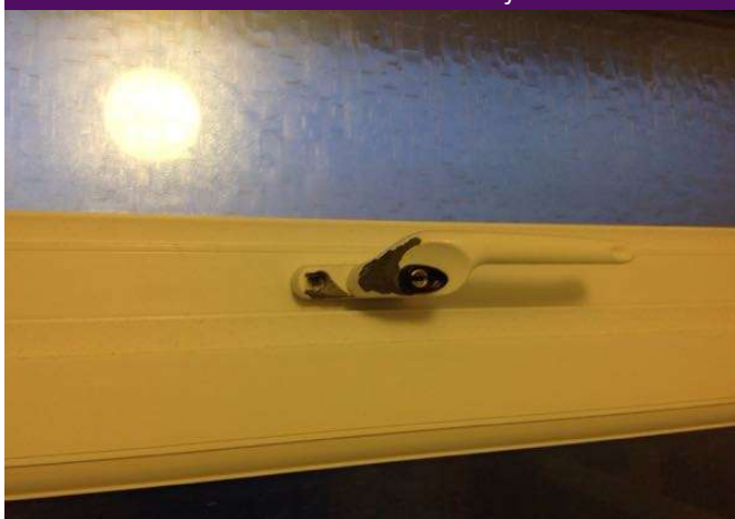
Handle broken on window
